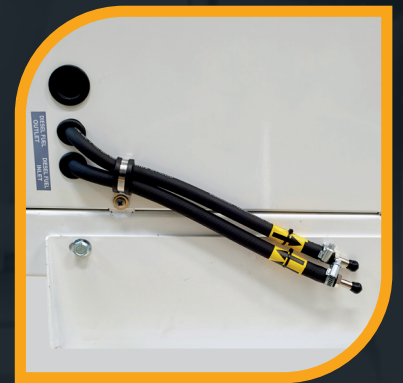
Fuel inlet and outlet
