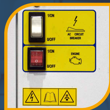
Main circuit breaker
