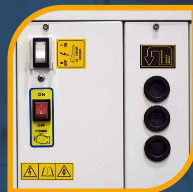
Main circuit breaker
