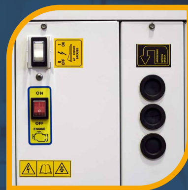
Main circuit breaker
