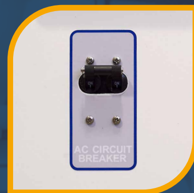
Main circuit breaker
