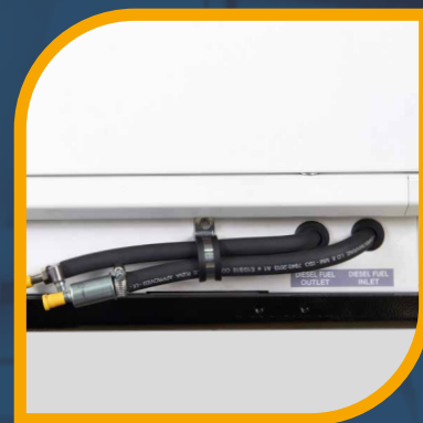
Input/Output fuel pipe
