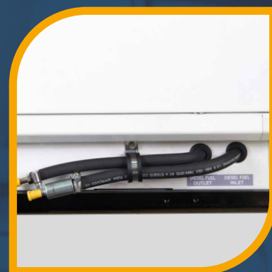
Input/Output fuel pipe
